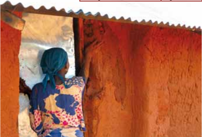
Shelters under construction in Dadaab. Much of the construction, including making mud blocks, is done by the women. Photo: Jake Zarins
